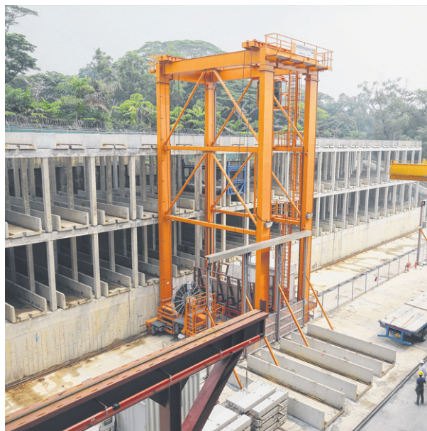
6 The completed component is removed from the mould and automatically transferred to the multi-storey precast storage rack.
