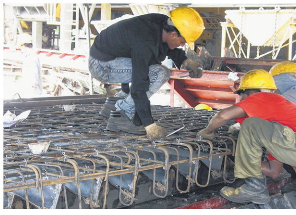
2 They fix steel wires known as rebars, to form the framework for casting.
