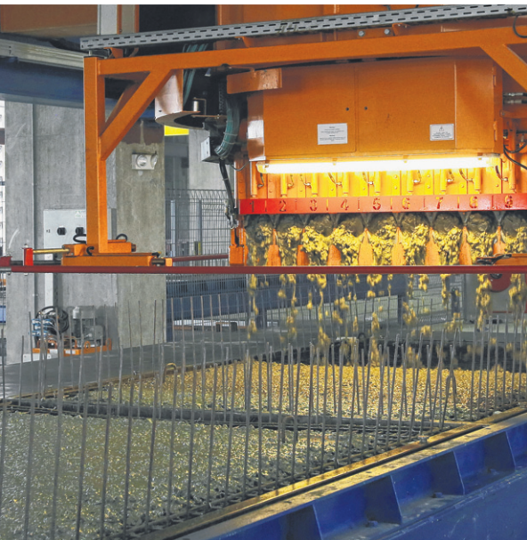
3 The mesh is placed inside the mould and concrete is poured in. The mould is vibrated by the machine to spread the concrete evenly.
