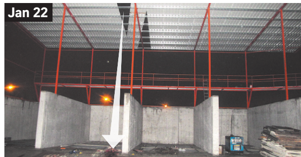
Jan 22 A construction worker fell 8.8m through a gap in the roof while laying zinc sheets.
