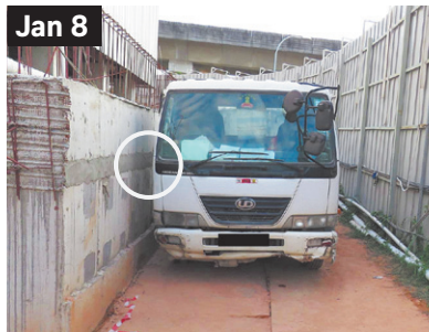
Jan 8 A construction worker was crushed when a truck rolled and trapped him against a wall.
