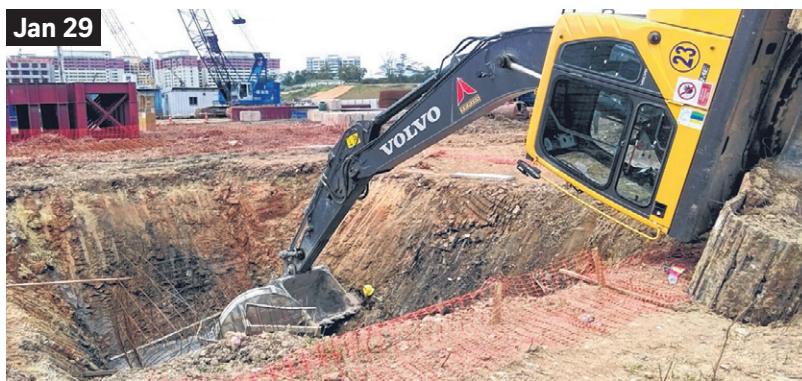
Jan 29 An excavator toppled into a pit at a worksite, injuring a construction worker with a concrete bucket it was carrying. He died later in hospital.
