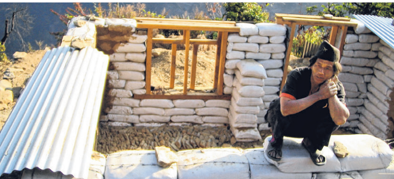
2. They are stacked on top of one another in a staggered fashion and held together by barbed wires. A trench is dug underground to form the foundation for the house.
