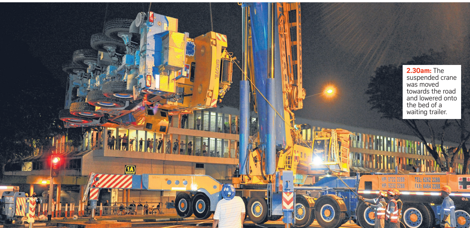
2.20am: The fallen crane was then hoisted and gingerly manoeuvred away from the building, freeing the crane's arm from the hole it had created in the wall of the bank.
